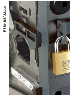
"Disconnected" position locking by padlocks.
